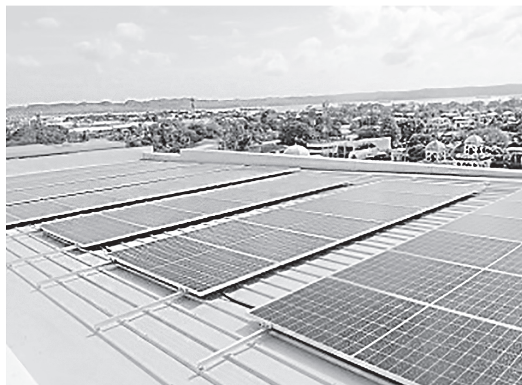
SOLAR POWER. Iloilo City Hall adopts solar energy. The power generated by the 134 solar panels is expected to generate 60 kilowatts a day and will provide around one-third of the power demand at the city hall. (PNA photo by PGLena)
