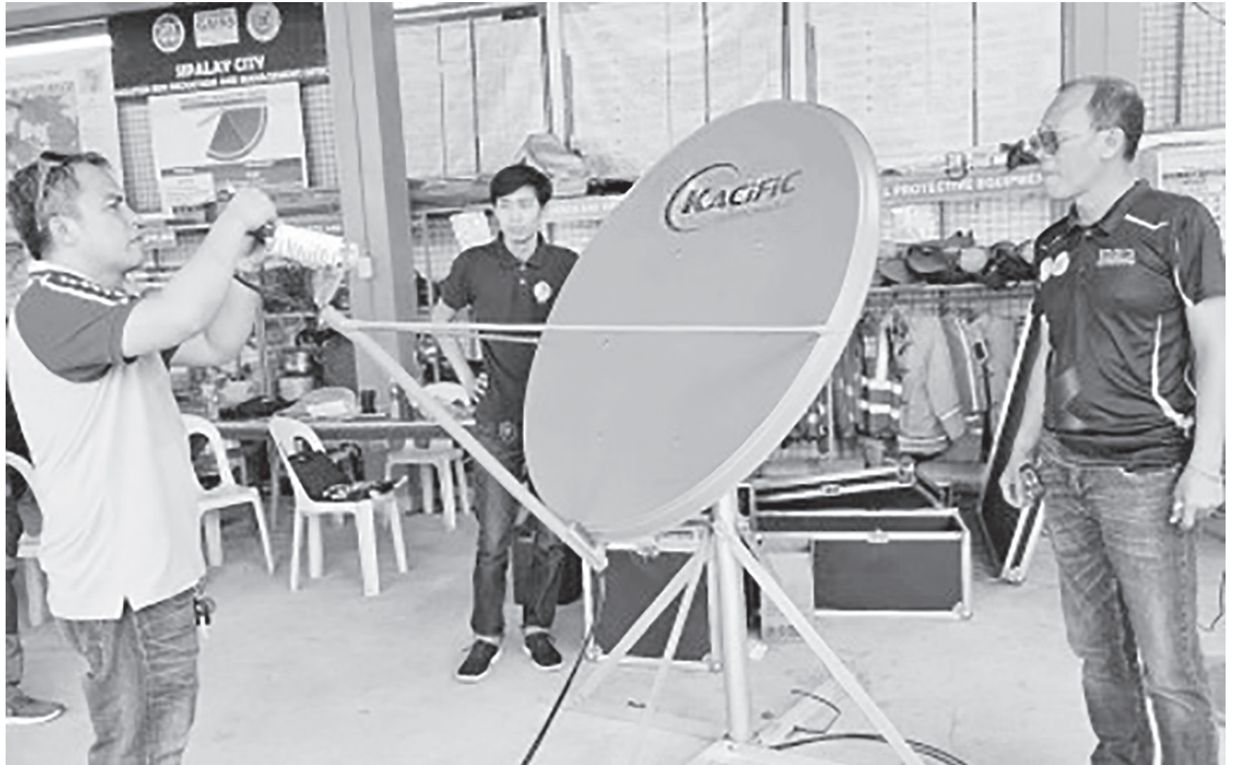
SATELLITE INTERNET. Department of Information and Communications Technology-Western Visayas Government Emergency Communications System personnel install the very small aperture terminal (VSAT) at the Sipalay City Disaster Risk Reduction and Management Operations Center on Jan. 23, 2024. Four disaster risk reduction and management offices in Negros Occidental are recipients of the VSAT satellite internet equipment from the Department of Information and Communications Technology. (Photo courtesy of Sipalay City-Local Government Unit)
