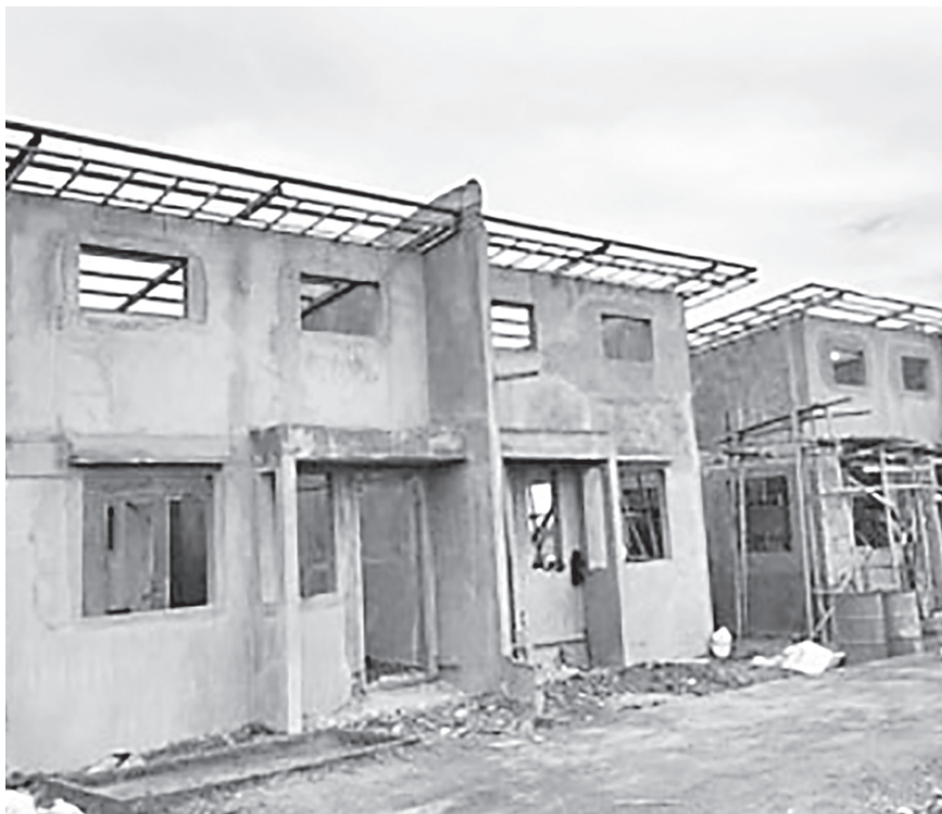
SHELTER PROJECT. The construction of the initial duplex-type units under the socialized housing project for government employees in Barangay 3 of Himamaylan City, Negros Occidental. The city government is proposing a collaboration with National Home Mortgage Finance Corp. to finance the ongoing development. (Photo from Mayor Raymund I. Tongson's Facebook page)
