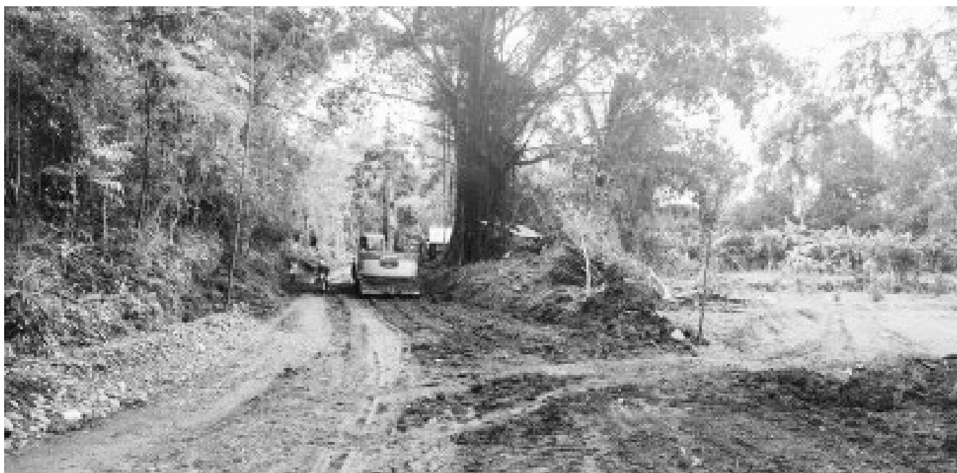
CONSTRUCTION. The construction of the PHP15 million farm-to-market road in San Jose de Buenavista starts on June 17, 2024. The project, once completed, will allow farmers easier access when bringing their produce to the market. (Photo courtesy of LGU San Jose de Buenavista)
