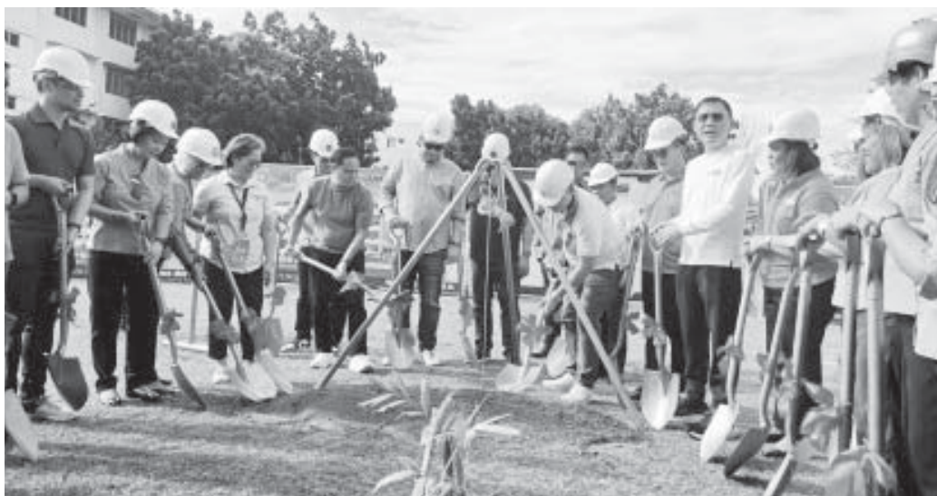
SCHOOL BUILDINGS PROJECT. Education Secretary Sonny Angara (6th from right) leads the simultaneous groundbreaking ceremony for the construction of school buildings in eight schools in the province at the Iloilo National High School in Iloilo City on Friday (Dec. 13, 2024). The projects are expected to be completed in time for the opening of the next school year. (PNA photo by PGLena)
