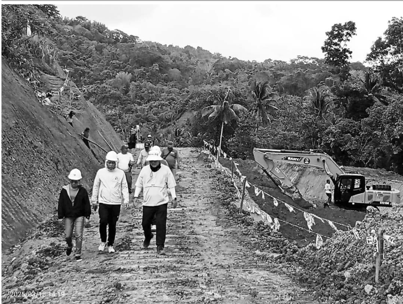
National Irrigation Administration (NIA) 6 Regional Manager and JRMP II Concurrent Project Manager Engineer Jonel B. Borresled the inspection of the Jalaur River Multi-purpose Project (JRMP) Stage II dams and High Line Canal even on March 18, 2025. He personally checked the status of water impounding in the High Dam and ongoing activities in the irrigation component of the project. Together with Manager Borres is the Division Manager for Construction Management, Engineer Gwendolyn Mae Velasco. (NIA 6)
